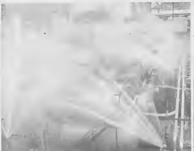
LIKE water, fire won't stop until it drowns itself. The fire-fighting equipment at the Acid Treatment Plant. The coverage of the installation is apparent in this picture of a "water" spread.
